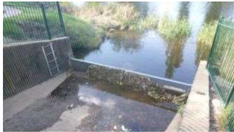
Trashrack (GPT) at Collett Street Queanbeyan
